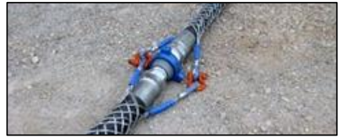
Figure 5 Hose to Hose
